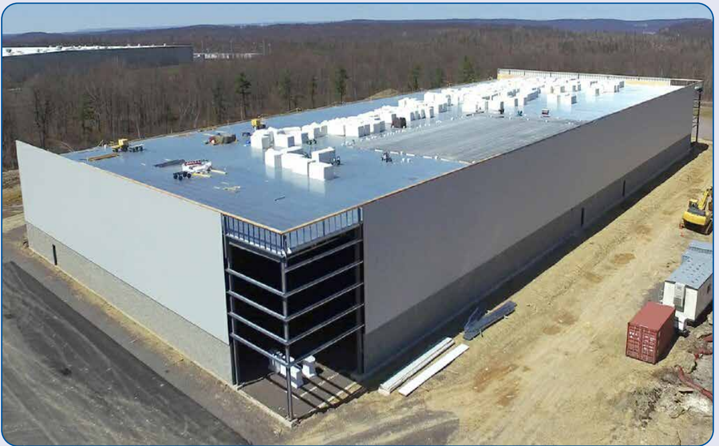
Tri-Mountain Realty leased its 70,000 square-foot facility, pictured here under construction, in Humboldt Industrial Park to Amazon.
